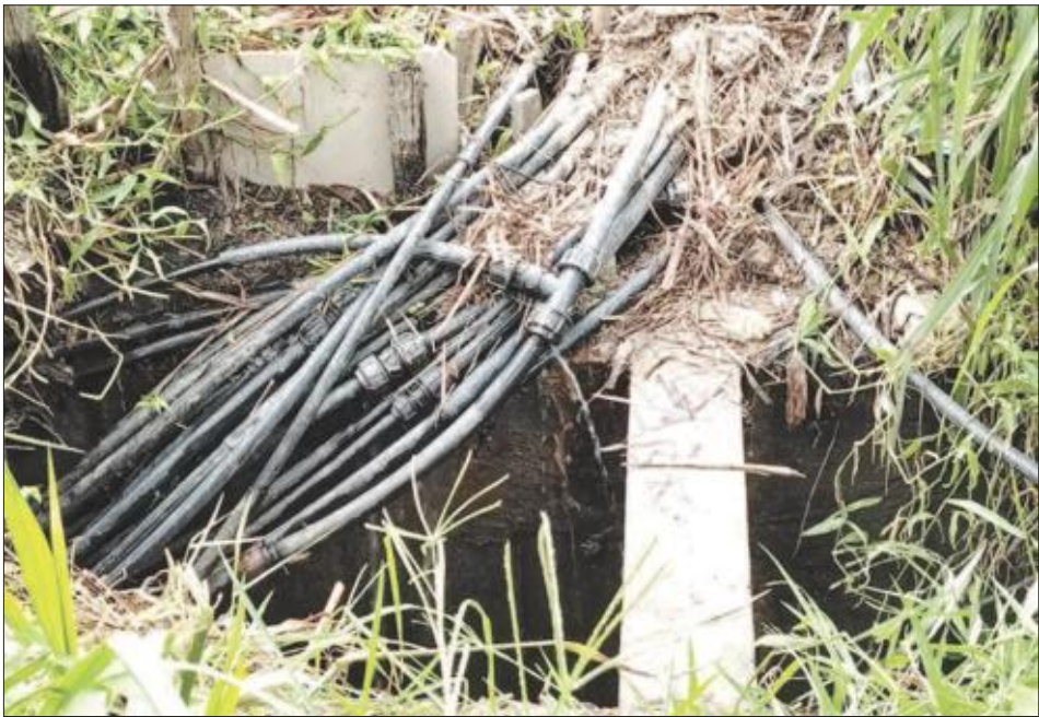
Some of the illegal water pipe connections cut off in Sandakan.
